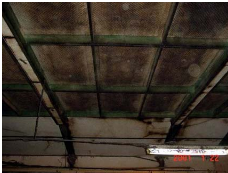
Figure 2. Porous ceiling inlet at the area of 300 m 2 (connection of porous ceiling with impermeable insulating panels PW3/A)
